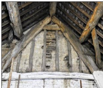
The cruck-framed Oak Fold Barn in Shiregreen, Sheffield, perhaps early 17th century with later alterations.
