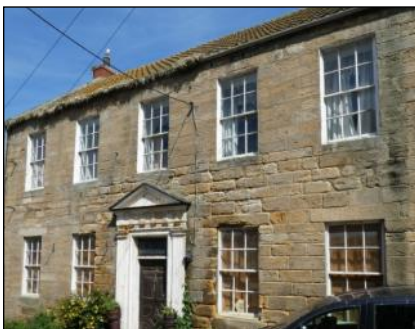
4. Kirkhill House (YVBSG 0925). Sadly, this house is now in need of some restoration. Likely built in the 1760s, the house was furnished with panelling, moulded door frames and a 'very fine' central staircase.
