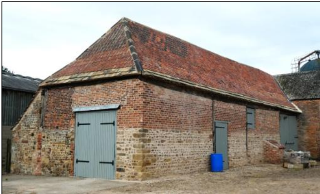
Nunwick House Farm barn, Nunwick (YVBSG 0045). Aisle on north side. Timberwork perhaps late sixteenth or early seventeenth century, with later walling.
