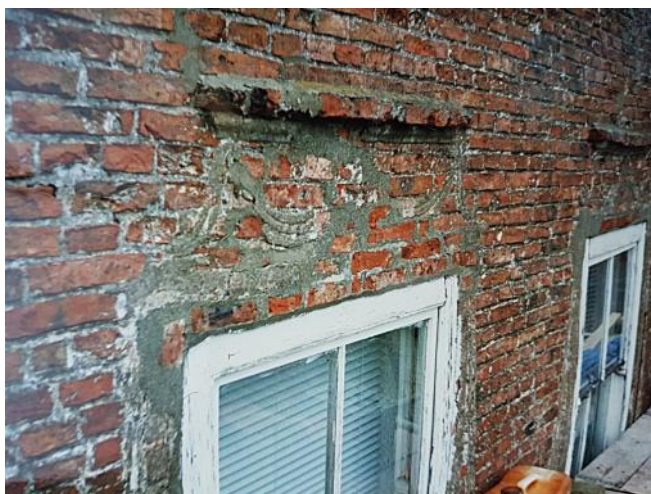
Remains of ornamental plasterwork under the drip moulds
