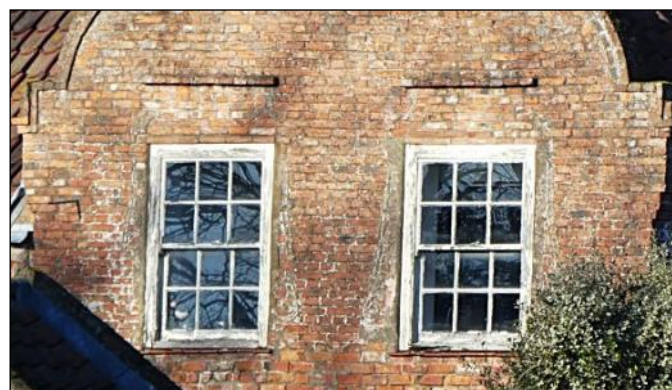
Rear gable as it appears today, photographed in 2025. The remains of scrolls are still visible down the sides of the sash windows.
