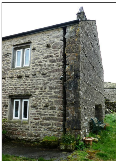
Weather wall at North Cote Farm. A gap of several inches has been left open between the weather wall and the gable wall of the house.
