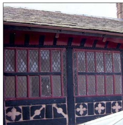
Decorated timber-framing hidden away at Rawcliffe Hall. Includes quatrefoils and coving under eaves.
