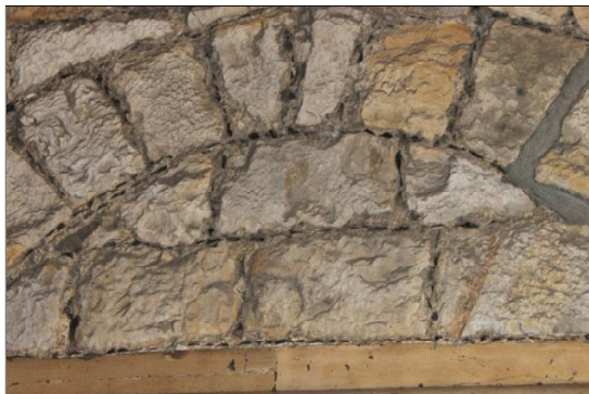
Fig 1. Early galleting – sixteenth century original?
