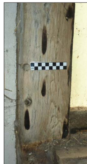
Burn marks at Bashall
